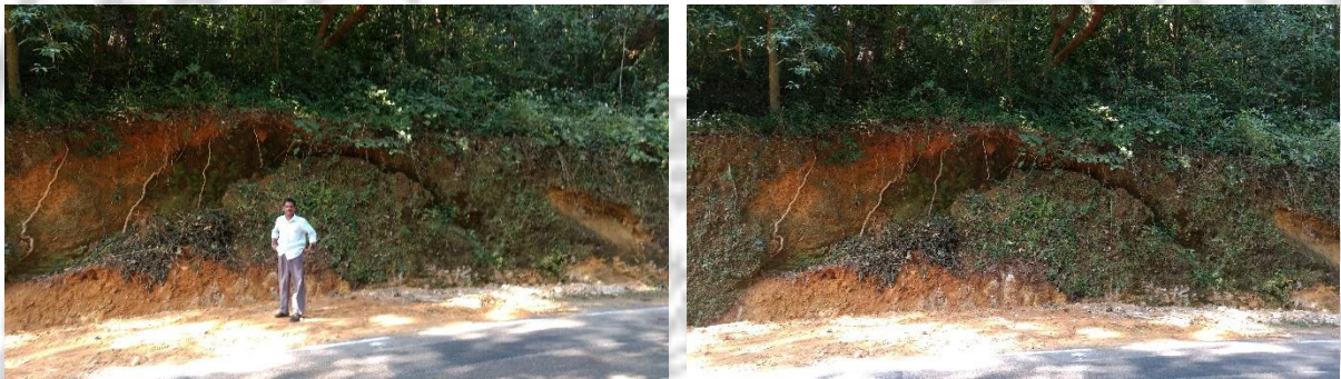
Photo: 2, Road cut failure due to toe disturbance.
